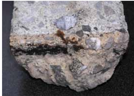
Fig. 4: Concrete core illustrating corrosion within carbonated zone
