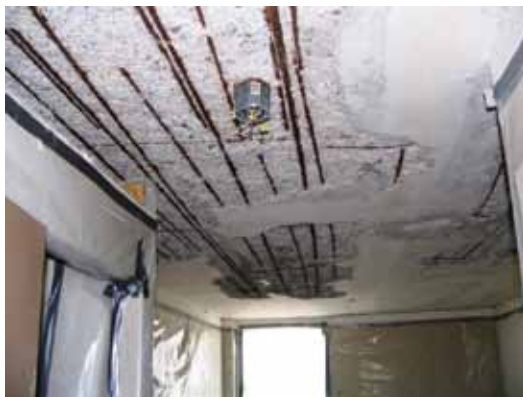
Fig. 2: Severe spalling of underside of roof slab
