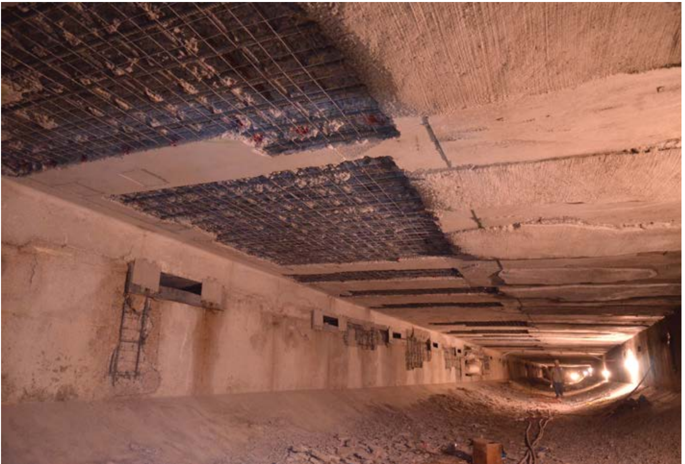
Fig. 4: Areas after hydrodemolition and hand chipping behind reinforcing steel ready for shotcrete
